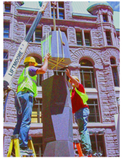
Install of Granite Columns in front of Minneapolis City Hall. 2 columns installed by St Cloud Granite at light rail station. Collaboration with Keith Christensen (2004)
